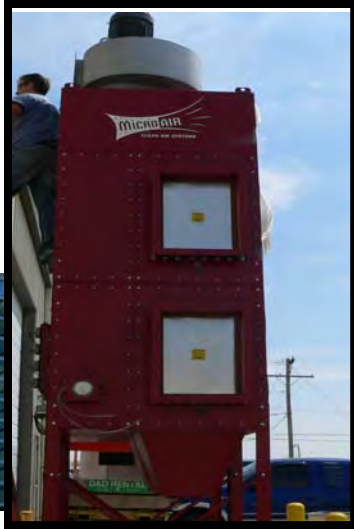
Micro Air RP8-2 Collector Equipped with Explosion Vents
